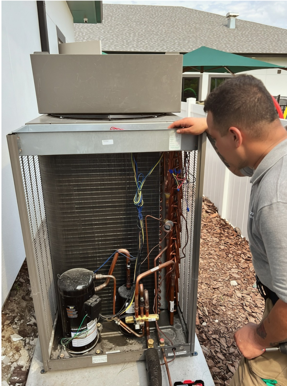
FIELD PHOTO 01 Inspecting an outdoor HVAC condenser and electrical connection points.
